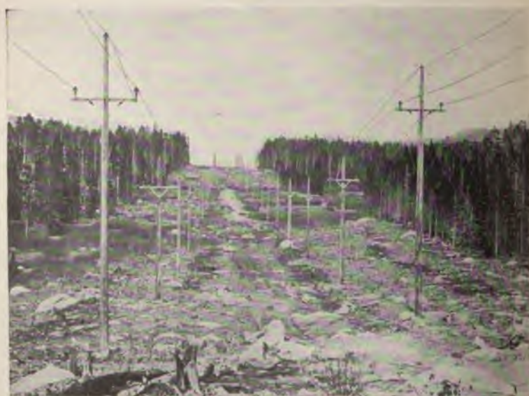
FIGS. 27 AND 28.—MISSOURI RIVER POWER COMPANY'S TRANSMISSION LINES.
